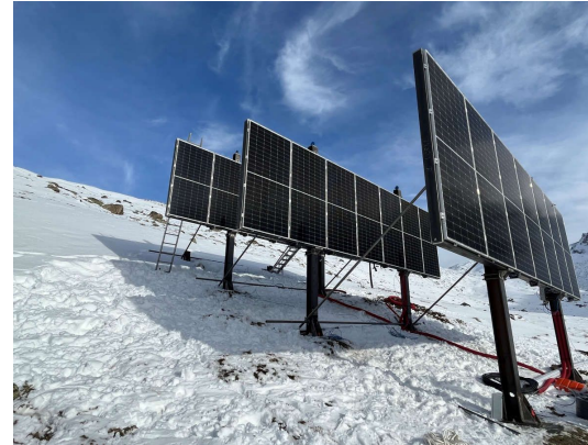
The test facility consists of three module tables, each with seven bifacial modules. (Vispताल Solar) Source: zvg
